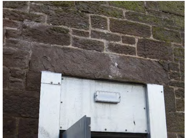
103 Spalling + cracking at lintel
