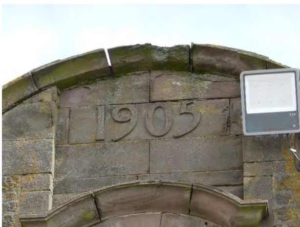
198 Cracked + delaminating at ornate masonry
