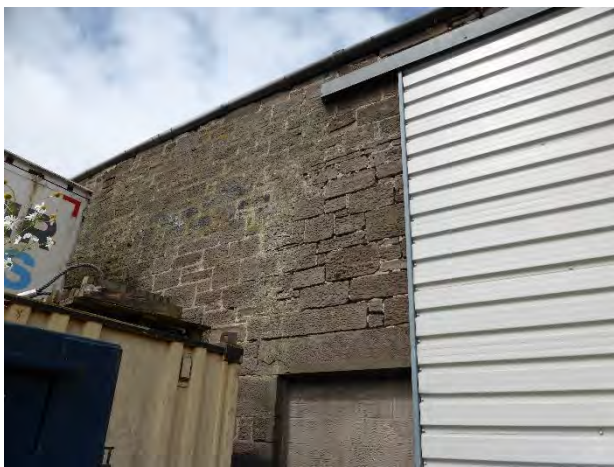
171 Failed pointing + open joints
