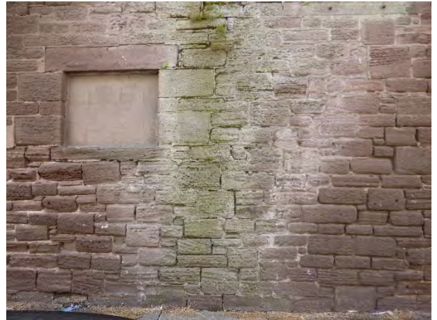
129 Algae + vegetation + stone decay + open joints
