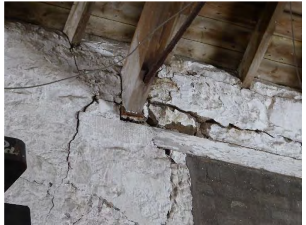
44 Cracks and loose masonry at rafter ends
