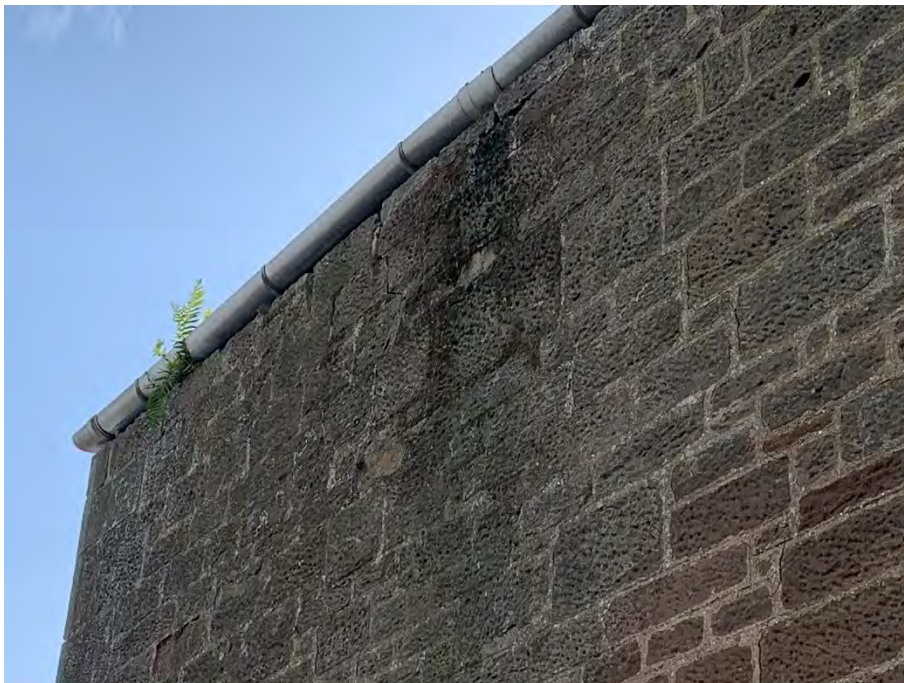
Figure 12: North East Elevation – Damp Patch, Weathered Stone ,Cracking & Gutter Position
