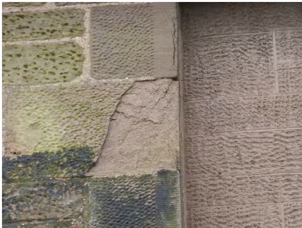
76 Surface loss + cracking at rybats
