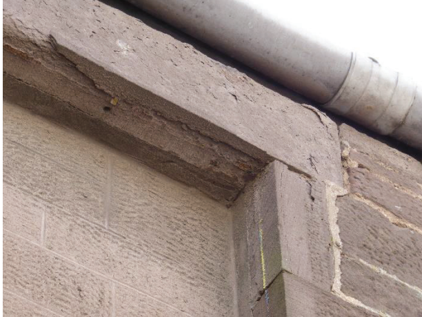
134 Spalling + cracking at lintel + rymat
