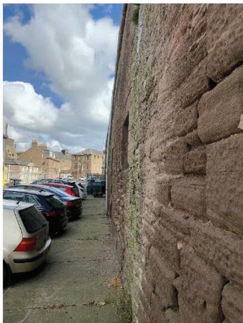
Figure 5: North West Elevation – Wall Lean
