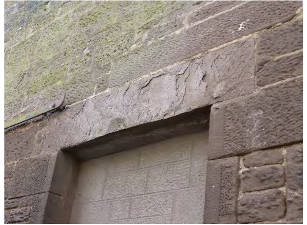
100 Spalling + cracking at lintel
