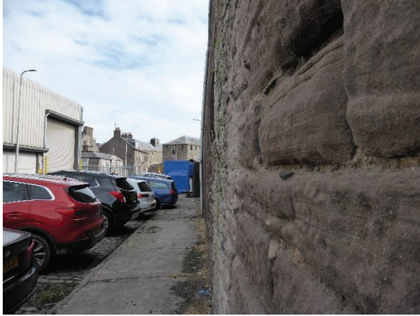
146 Bowed wall leaning into street
