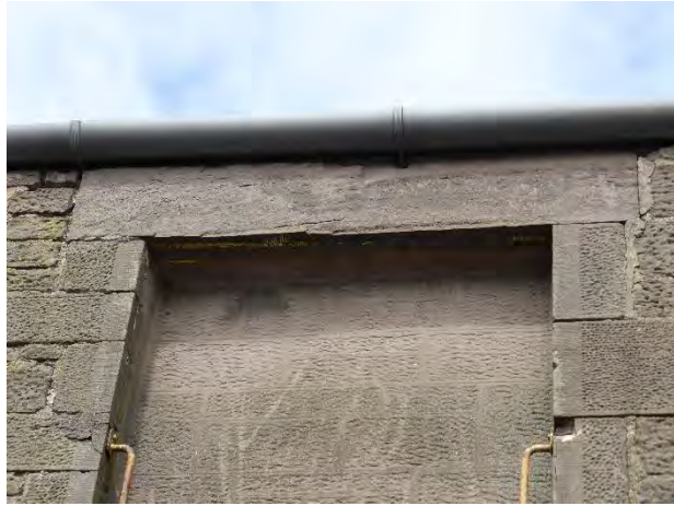
180 Cracked + spalling lintel + cracked rybats
