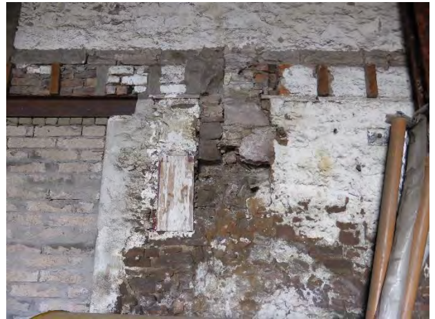
29 Crude repairs + pockets of missing rubble
