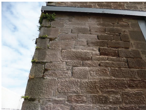
209 Stone decay + open joints + vegetation
