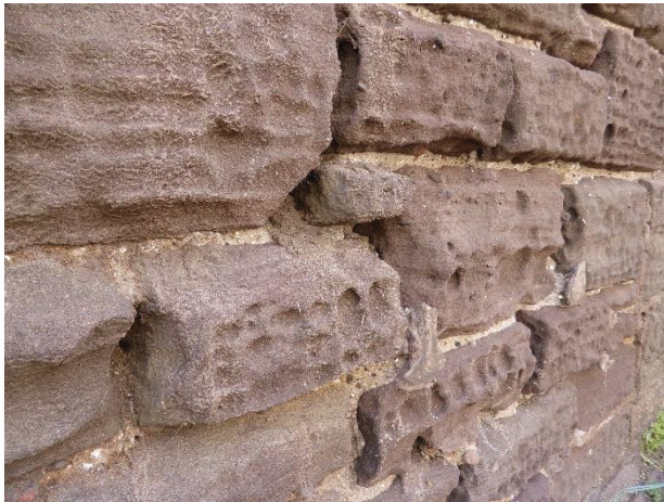
138 Stone decay + open joints
