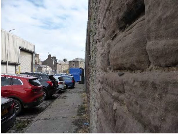
146 Bowed wall leaning into street
