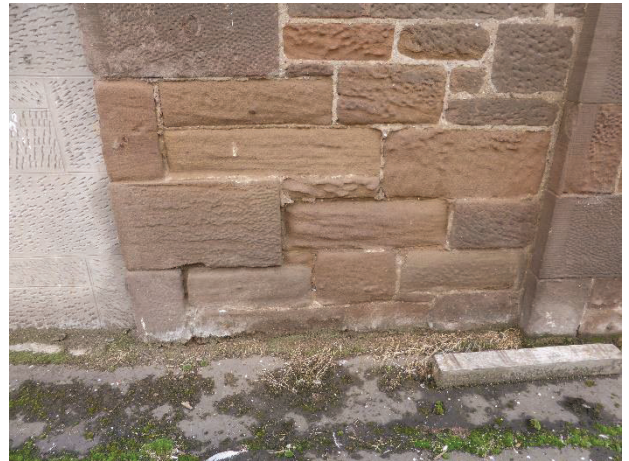
71 Stone decay + open joints
