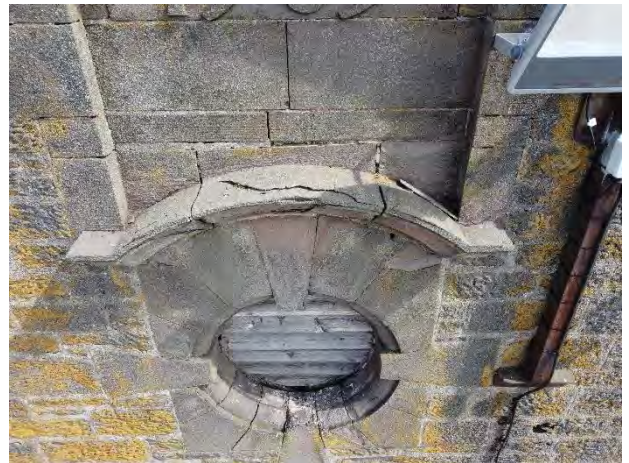
23 Cracked + delaminating at ornate masonry
