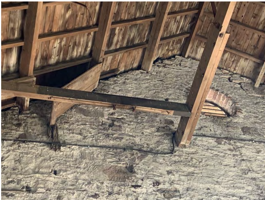
Figure 14: Internal South West Elevation –Weathered Stone & Cracking, Truss Discolouring
