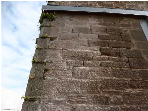
209 Stone decay + open joints + vegetation
