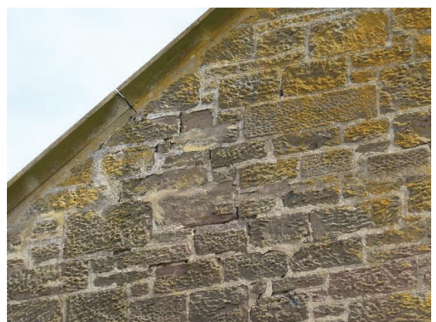
200 Stone decay + open joints
