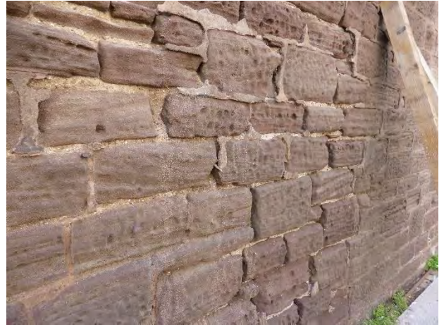
137 Stone decay + open joints
