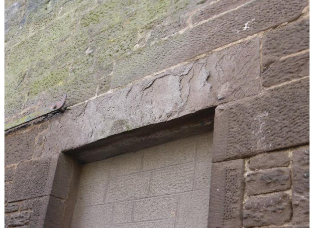
100 Spalling + cracking at lintel
