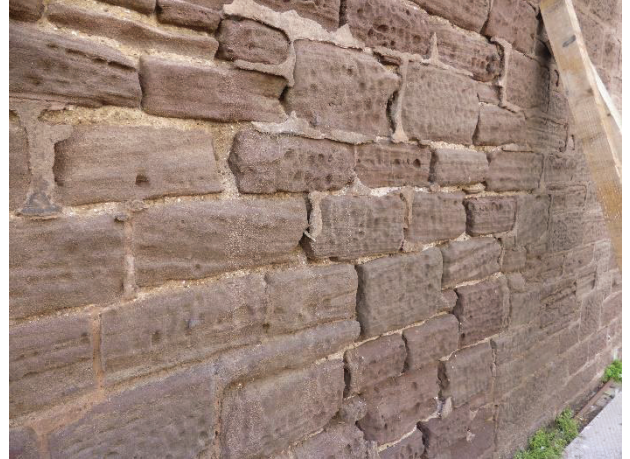
137 Stone decay + open joints
