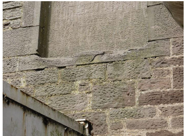
177 Delaminating + spalling sill
