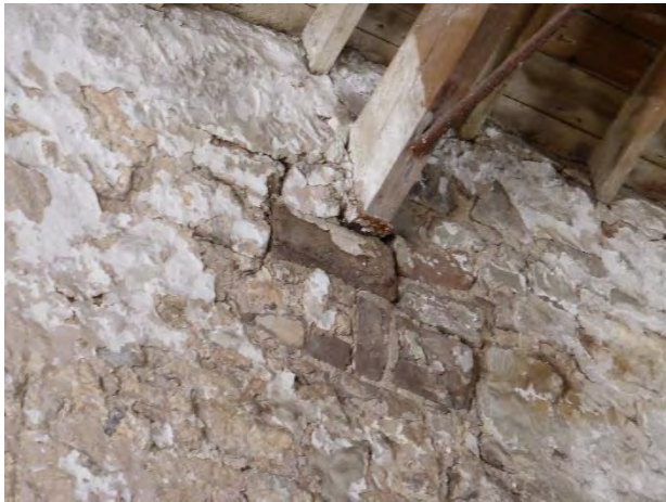
43 Cracks and loose masonry at rafter ends
