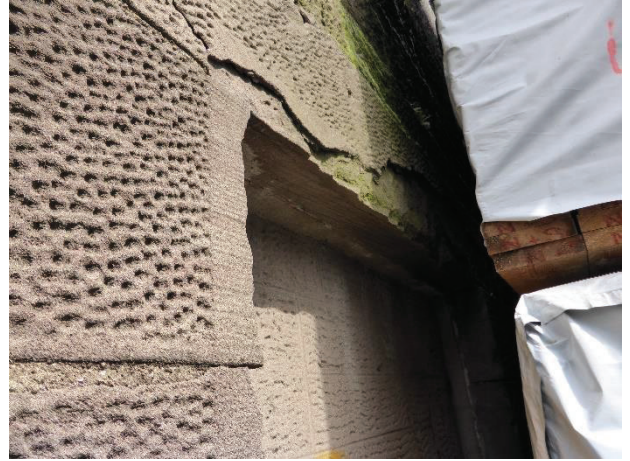
166 Cracked + spalling lintel
