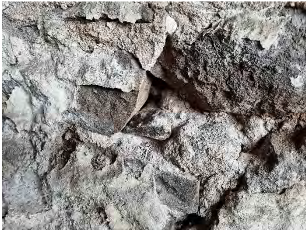
1 Loose + missing rubble
