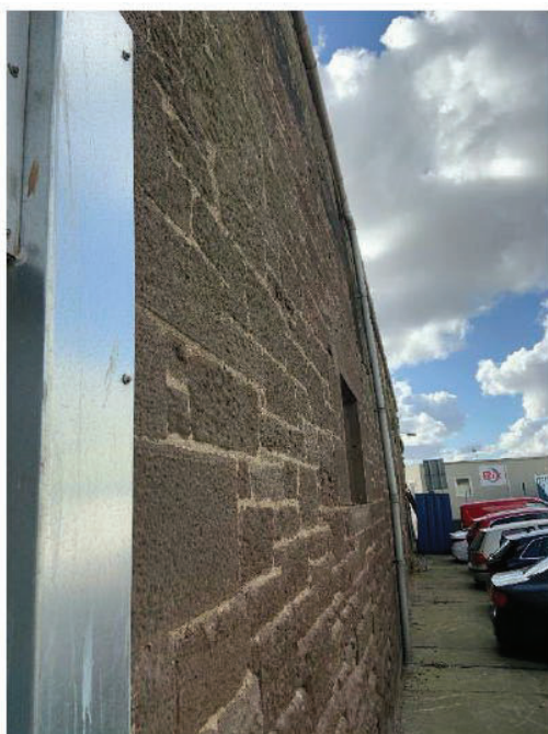
Figure 6: North West Elevation – Wall Lean
