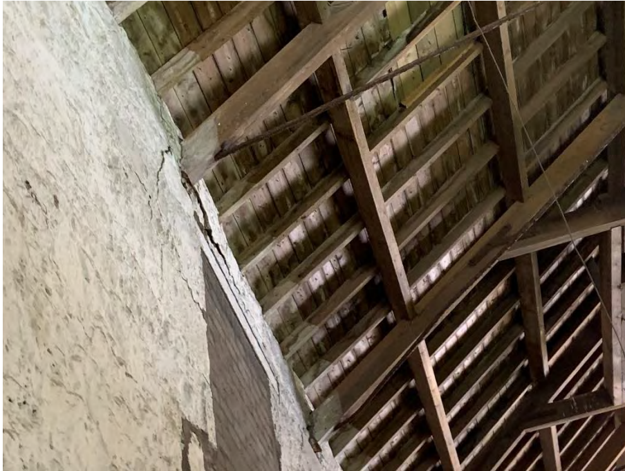
Figure 19: Internal North East Elevation –Wall Lean, Wall Displacement, Patches & Cracking
