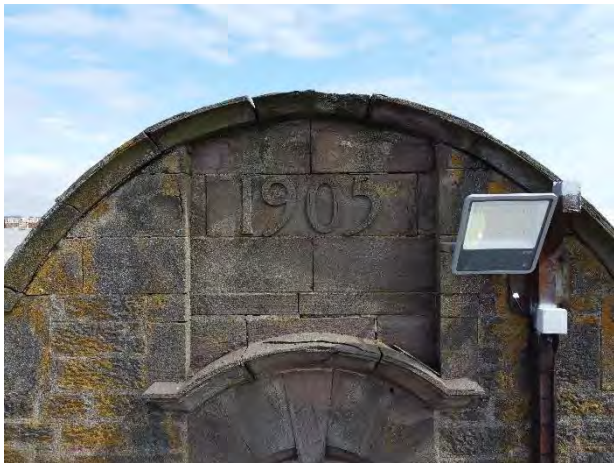
20 Cracked + delaminating at ornate masonry
