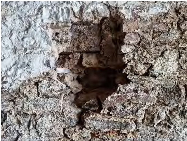
4 Loose + missing rubble
