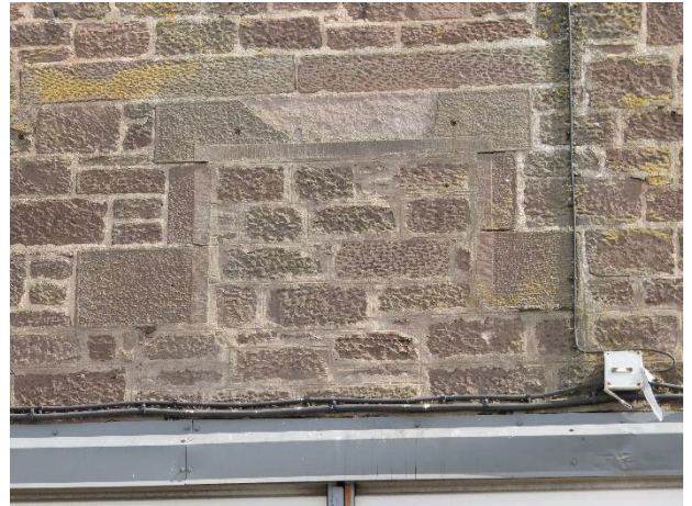
202 Spalling at lintel
