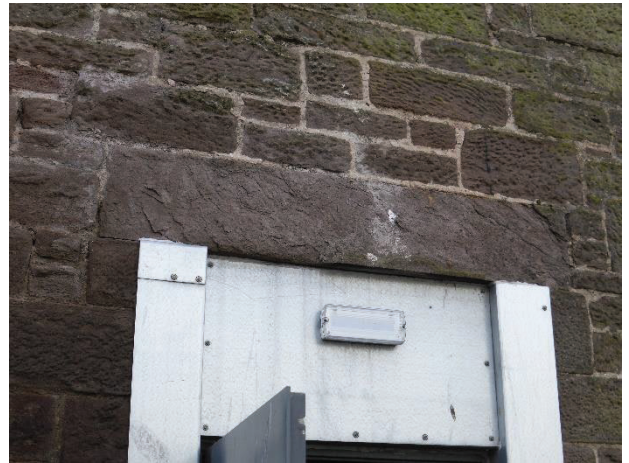
103 Spalling + cracking at lintel
