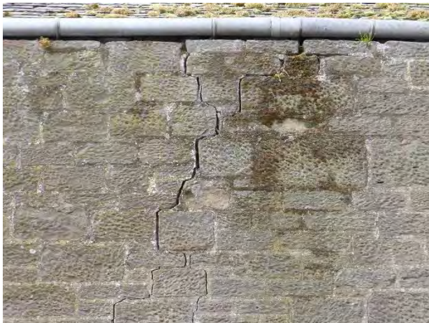
154 Structural movement cracks
