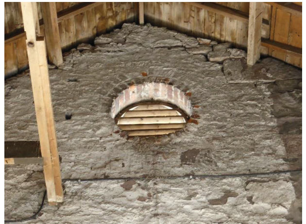
50 Cracks and loose masonry at purlin ends
