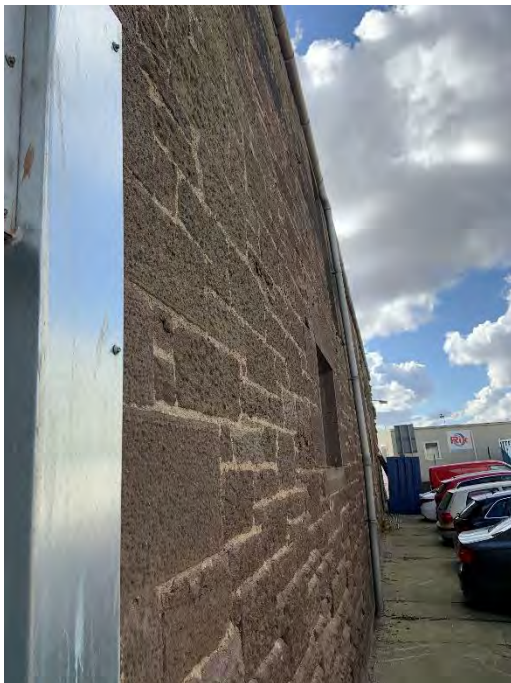
Figure 6: North West Elevation – Wall Lean
