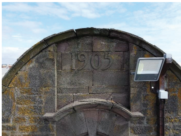
20 Cracked + delaminating at ornate masonry
