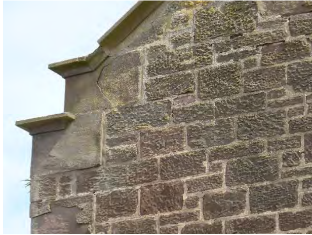
201 Stone decay + spalling at quoins
