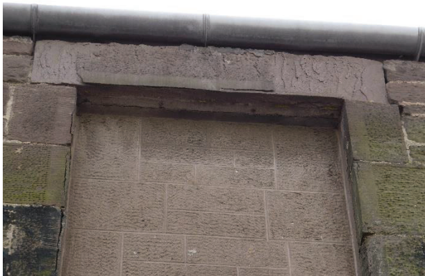
91 Spalling + cracking at lintel
