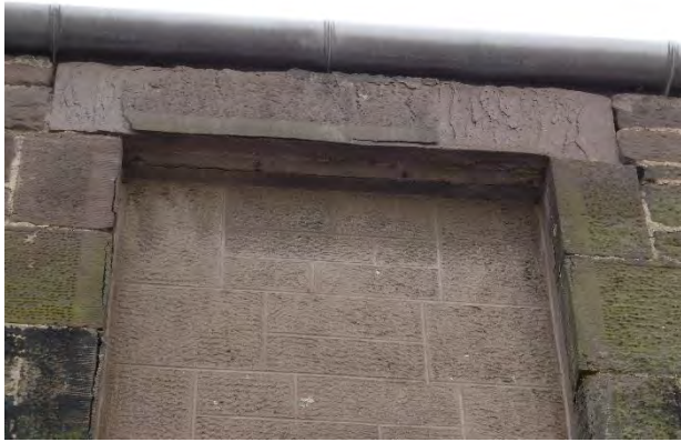
91 Spalling + cracking at lintel
