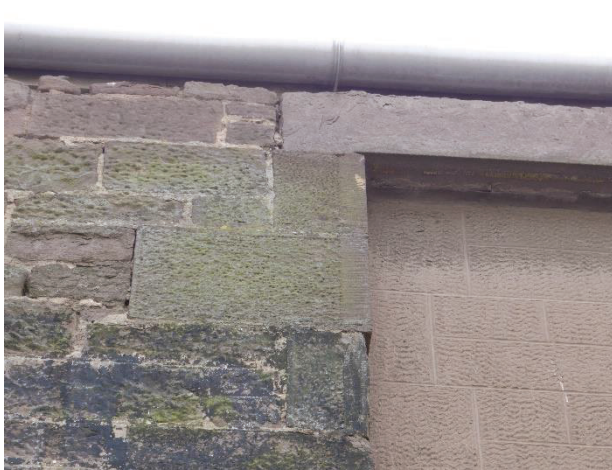
112 Spalling + cracking at lintel
