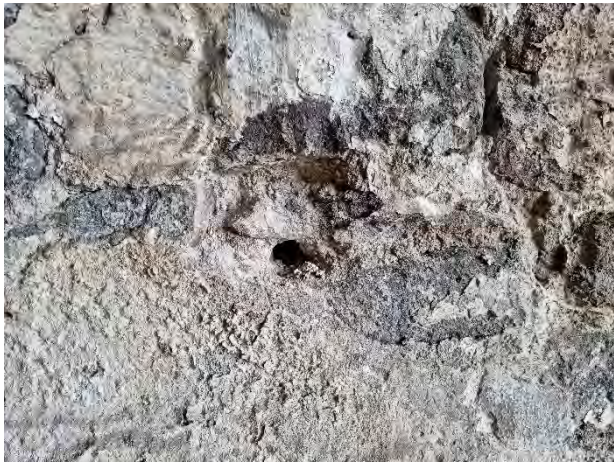
2 Loose + missing rubble
