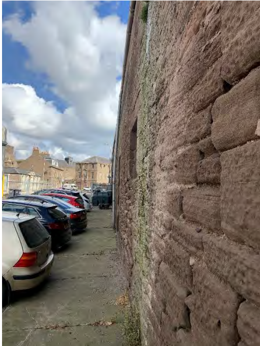
Figure 5: North West Elevation – Wall Lean
