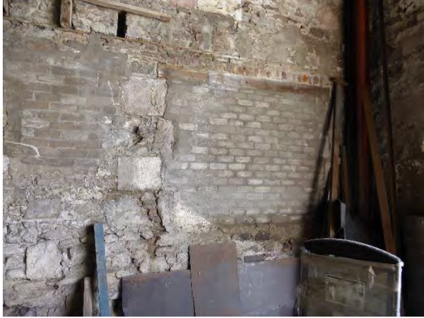
16 Crude repairs + pockets of missing rubble
