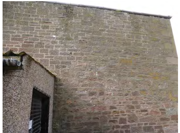
150 Structural movement cracks
