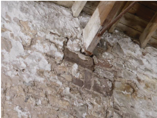
43 Cracks and loose masonry at rafter ends
