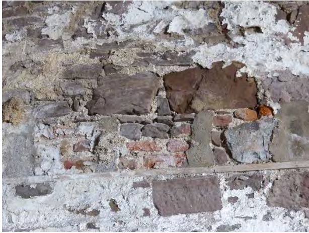
36 Loose and friable mortar pointing
