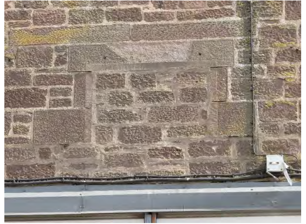
202 Spalling at lintel
