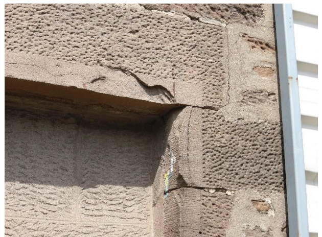
220 Cracked lintel + rybats
