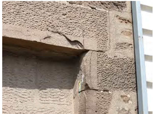
220 Cracked lintel + rybats
