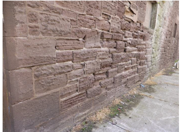
121 Stone decay + open joints
