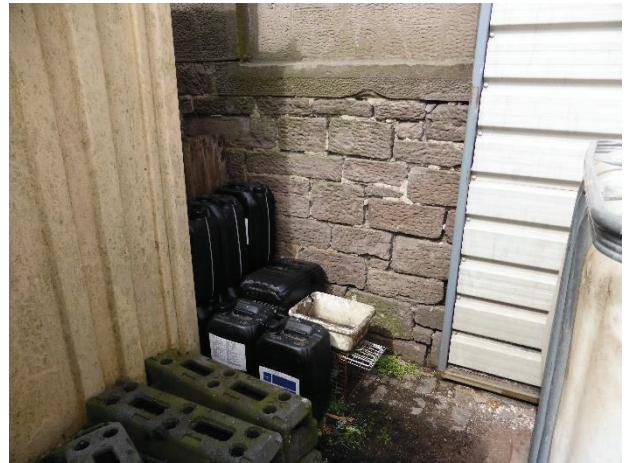
172 Failed pointing + open joints
