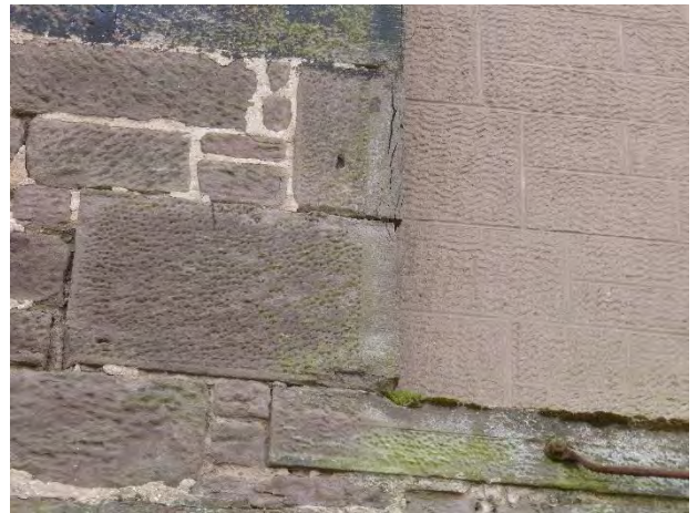
111 Cracking at rybats
