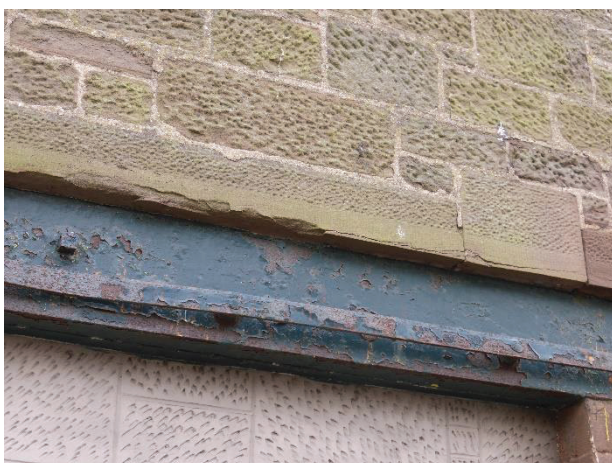
82 Delaminating lintel course
