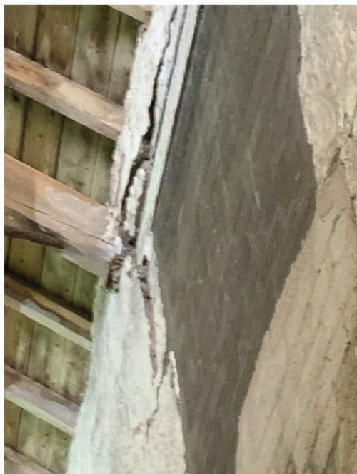
Figure 20: Internal North East Elevation –Wall Leam, Wall Displacement, Patches & Cracking
