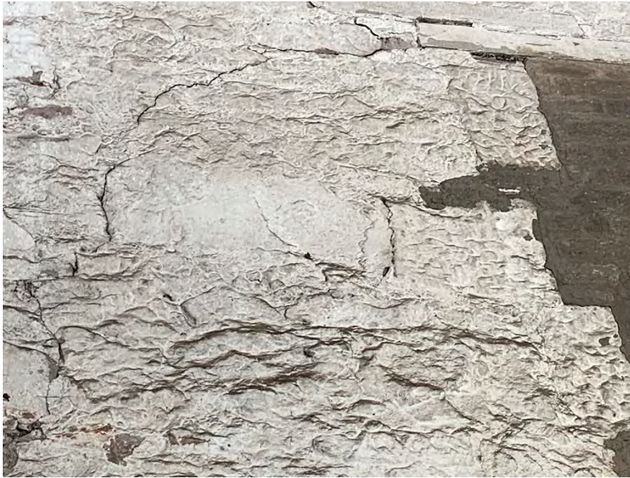
Figure 23: Internal North East Elevation –Diagonal Crack
