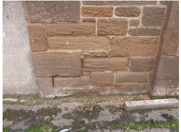
71 Stone decay + open joints
