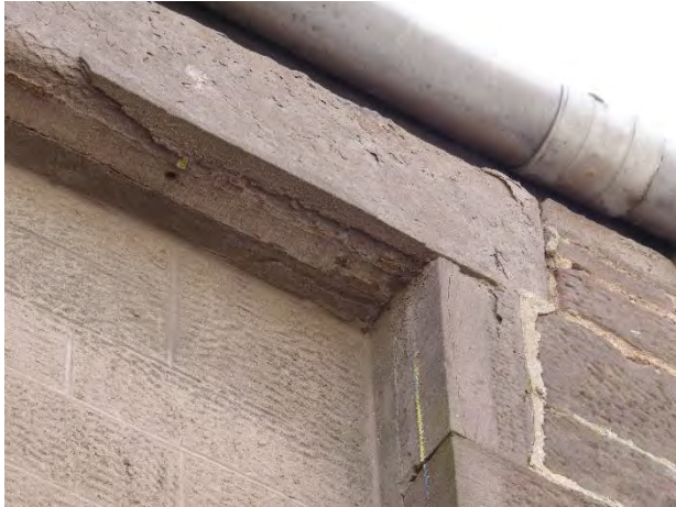
134 Spalling + cracking at lintel + rymat
