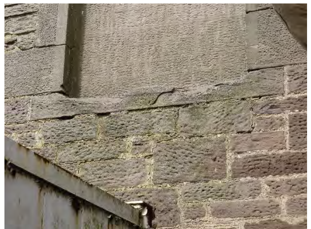
177 Delaminating + spalling sill
