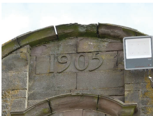
198 Cracked + delaminating at ornate masonry
