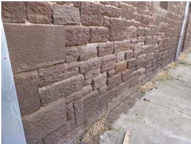
106 Stone decay + open joints
