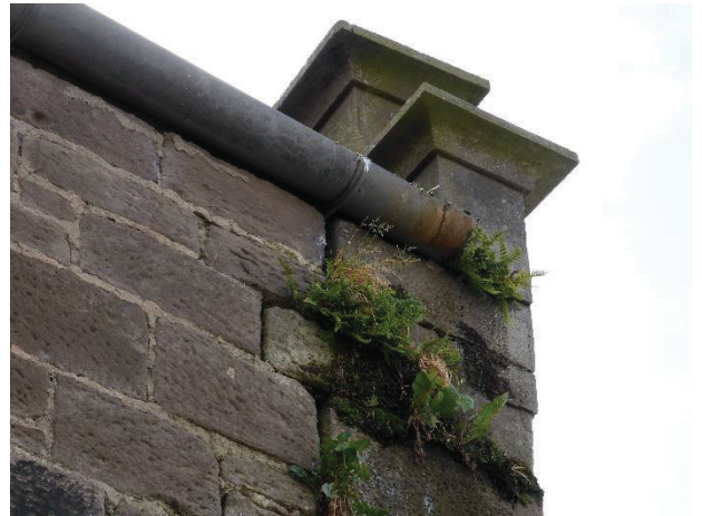
Structural movement + widened joints
