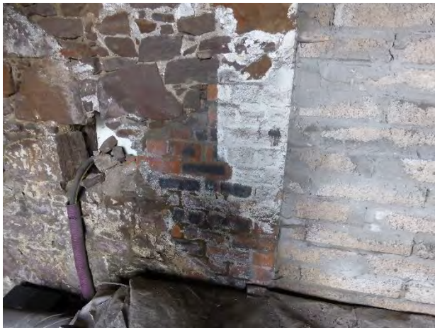
31 Crude repairs + hole through wall
