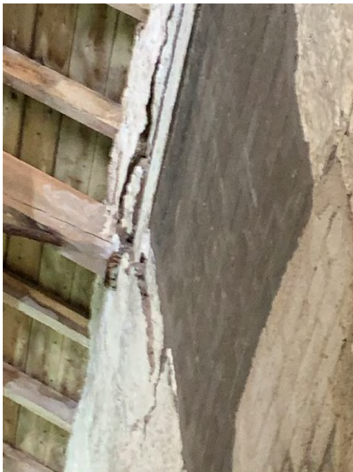
Figure 20: Internal North East Elevation –Wall Lean, Wall Displacement, Patches & Cracking
