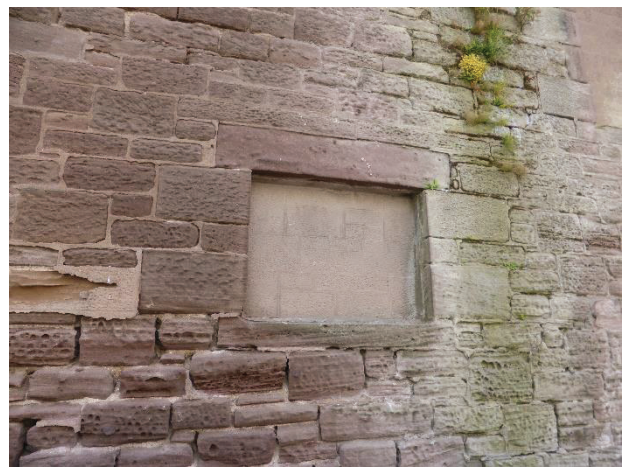
124 Stone decay + open joints
