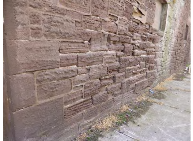
121 Stone decay + open joints
