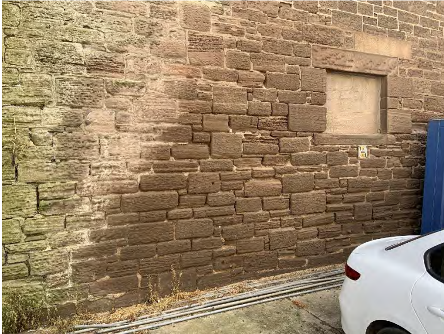
Figure 7: North West Elevation – Damp Patch, Weathered Stone & Eroded Friable Mortar
