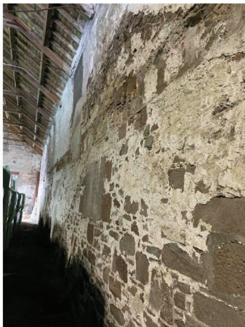
Figure 17: Internal South West Elevation –Wall Leam, Weathered Stone, Patches & Cracking
