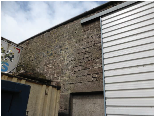
171 Failed pointing + open joints
