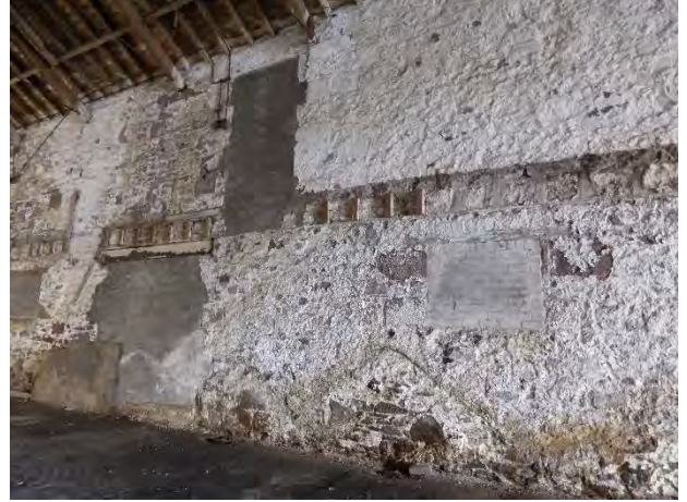
19 Crude repairs + pockets of missing rubble
