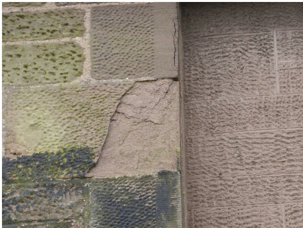
76 Surface loss + cracking at rybats
