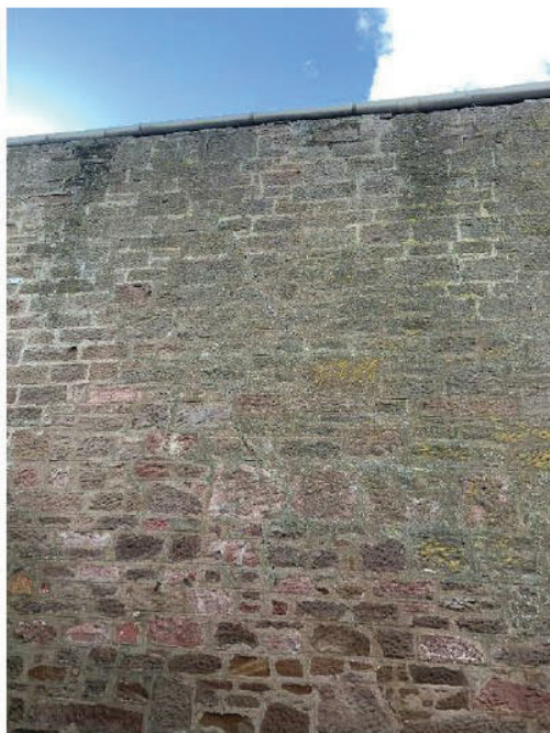
Figure 9: North East Elevation – Damp Patch, Weathered Stone & Cracking
