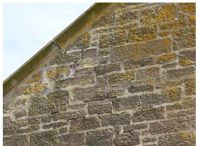
200 Stone decay + open joints
