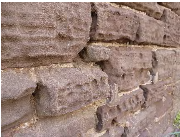
138 Stone decay + open joints
