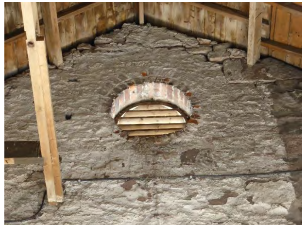
50 Cracks and loose masonry at purlin ends
