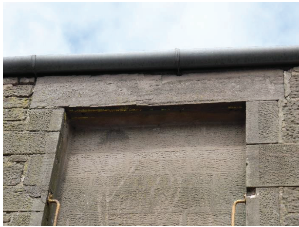
180 Cracked + spalling lintel + cracked rybats
