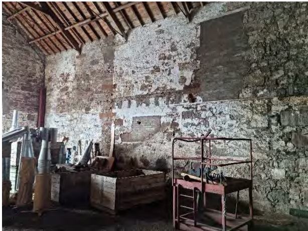
6 Crude repairs + pockets of missing rubble
