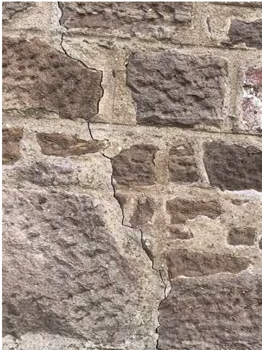
Figure 10: North East Elevation – Typical Crack
