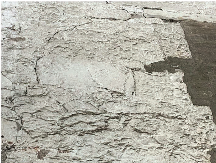
Figure 23: Internal North East Elevation –Diagonal Crack
