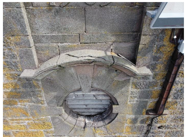
23 Cracked + delaminating at ornate masonry
