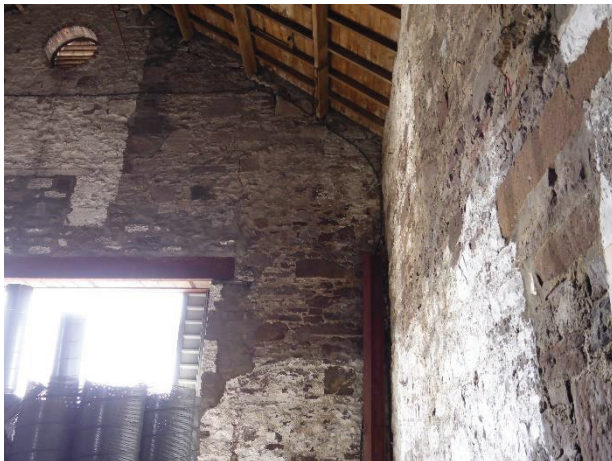
48 Vertical crack through rubble to right side
