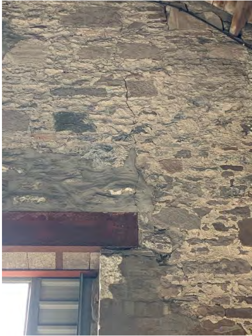
Figure 15: Internal South West Elevation –New Lintel with Vertical Crack
