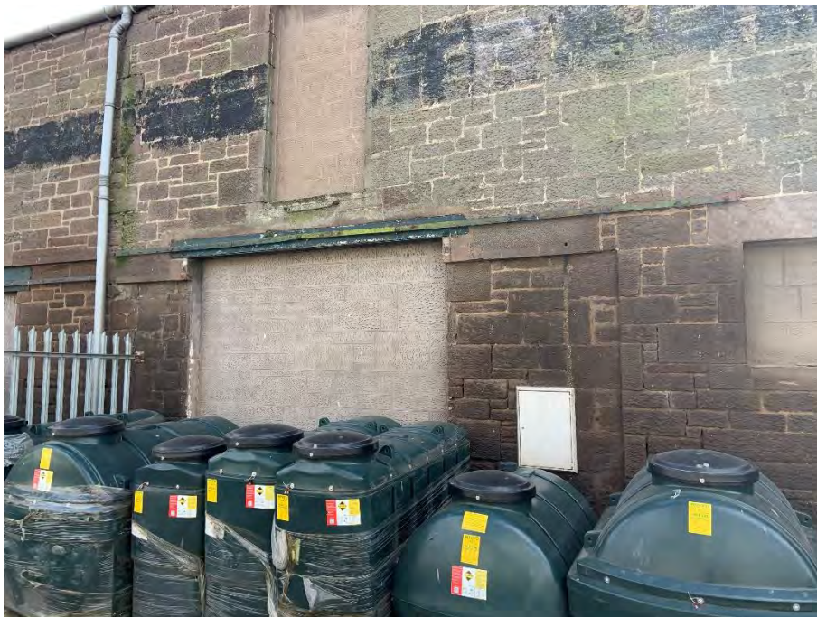
Figure 8: North West Elevation – Altered Openings, Damp Pathces & Eroded Stone and Mortar
