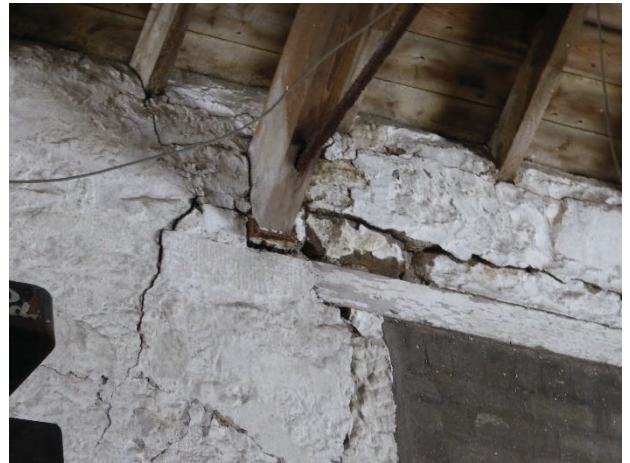
44 Cracks and loose masonry at rafter ends
