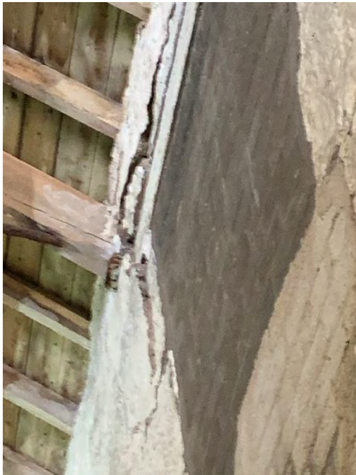
Figure 18: Internal North East Elevation –Wall Lean, Wall Displacement, Patches & Cracking
