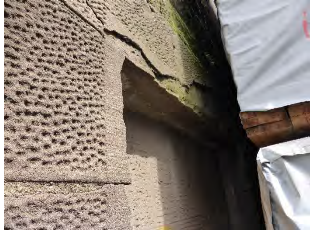
166 Cracked + spalling lintel
