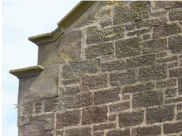
201 Stone decay + spalling at quoins
