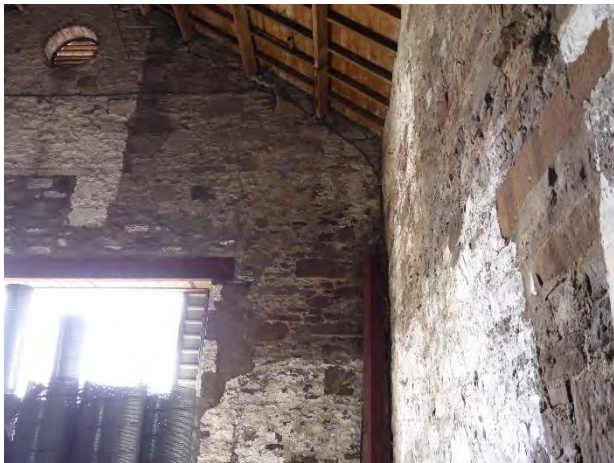
48 Vertical crack through rubble to right side
