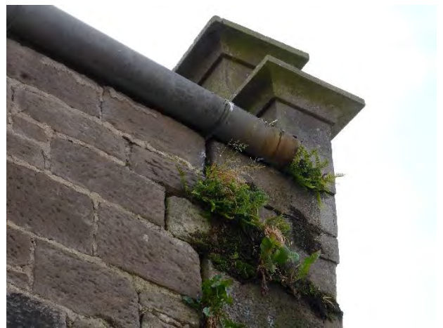
Structural movement + widened joints
