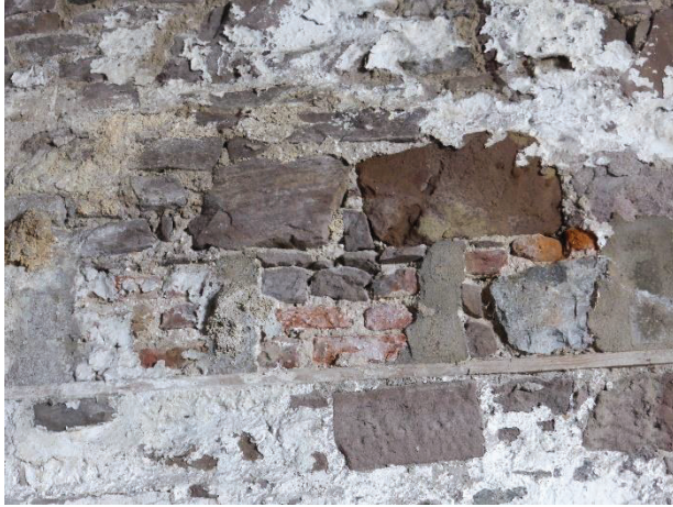
36 Loose and friable mortar pointing
