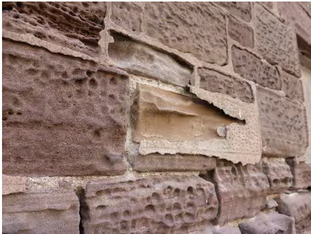
122 Stone decay + open joints
