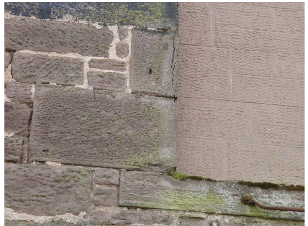
111 Cracking at rybats
