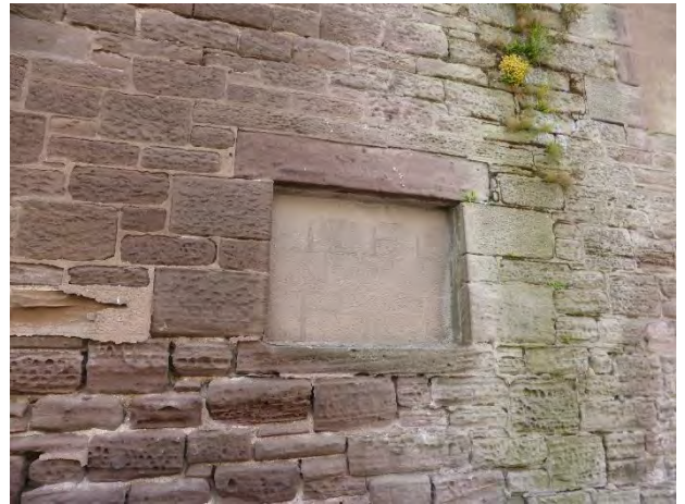
124 Stone decay + open joints
