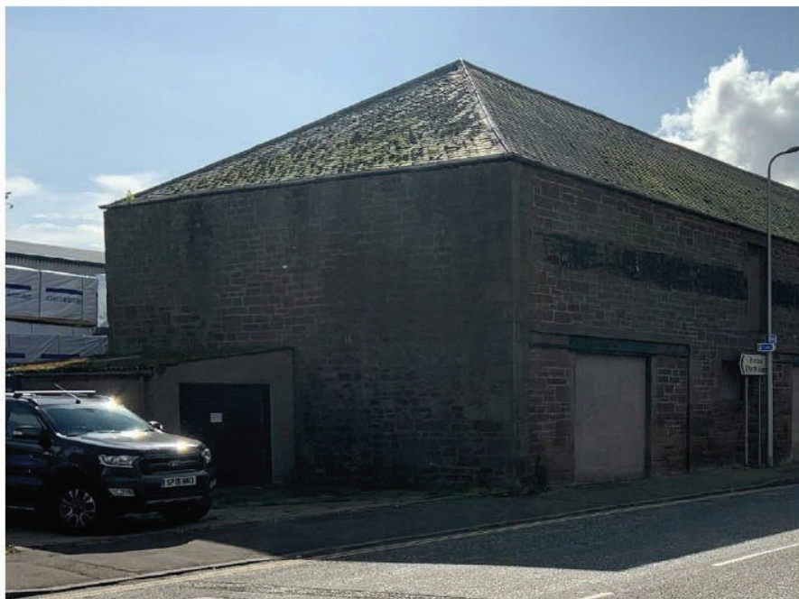
Figure 13: North East Elevation – Wall off Plumb (Left Hand Corner)
