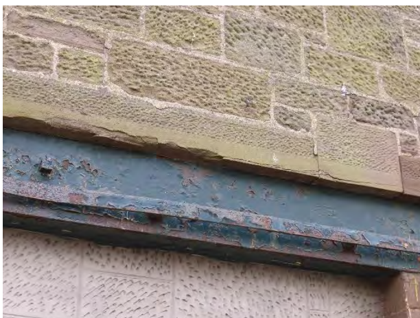
82 Delaminating lintel course
