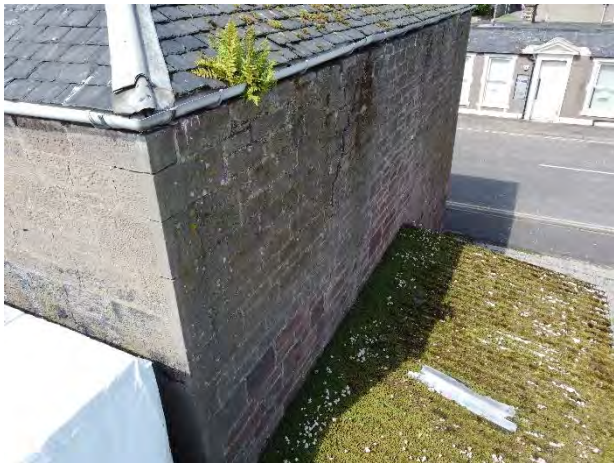
48 Outwards leaning of the wall
