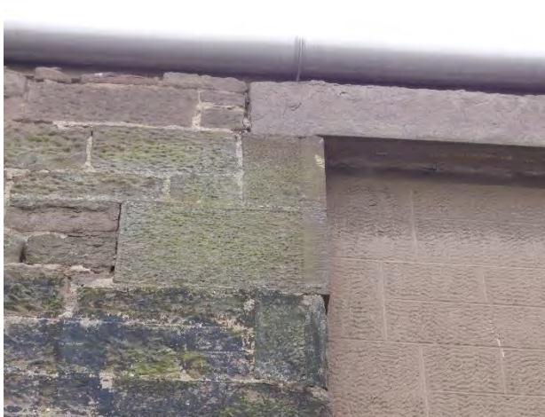
112 Spalling + cracking at lintel
