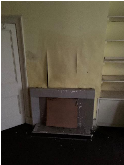
Photograph 1.09 Managers House - Internal Wall Fireplace & Dampness
