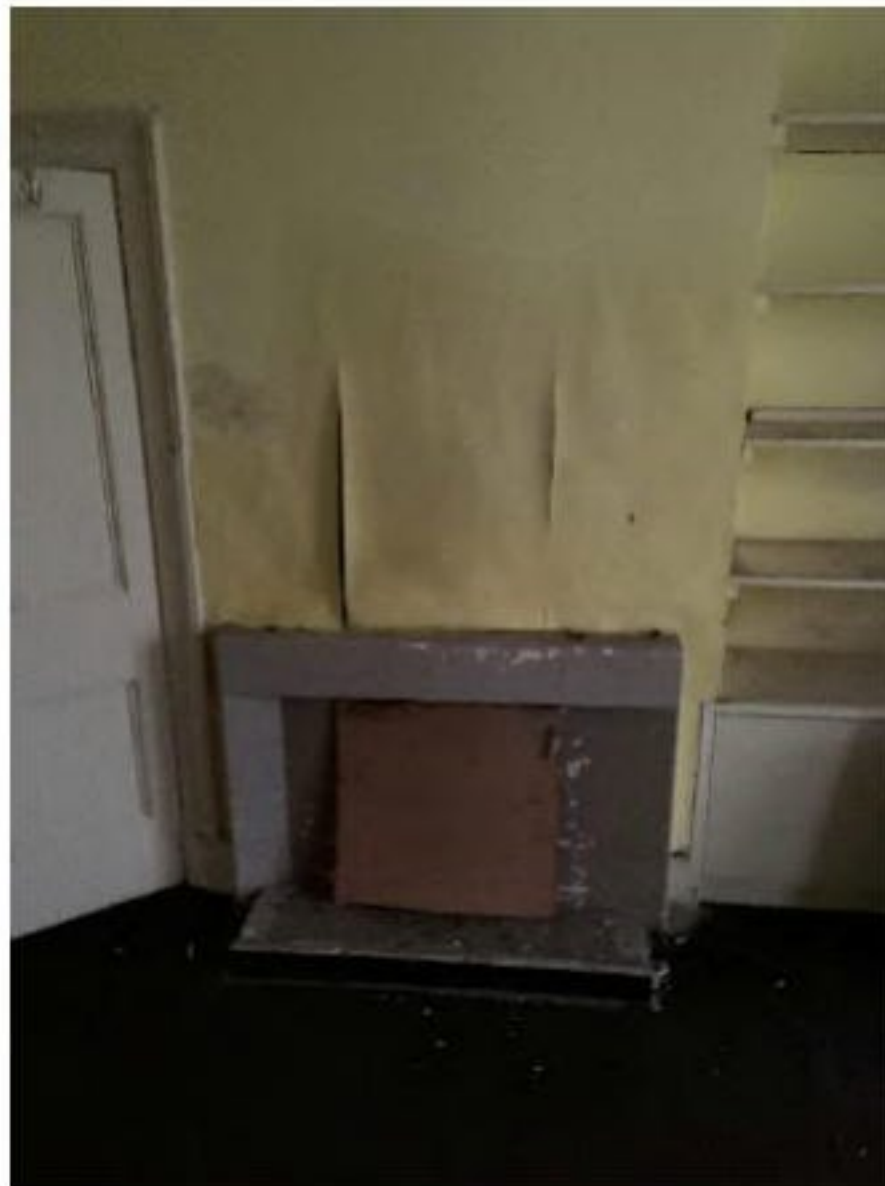
Photograph 1.09 Managers House - Internal Wall Fireplace & Dampness
