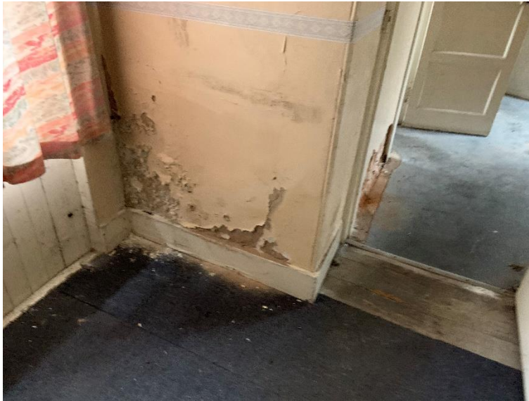
Photograph 1.08 Managers House - Internal Wall Dampness
