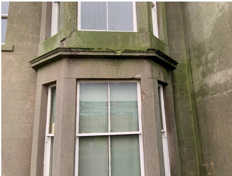
Photograph 1.03 Managers House - External Wall - Crack 2
