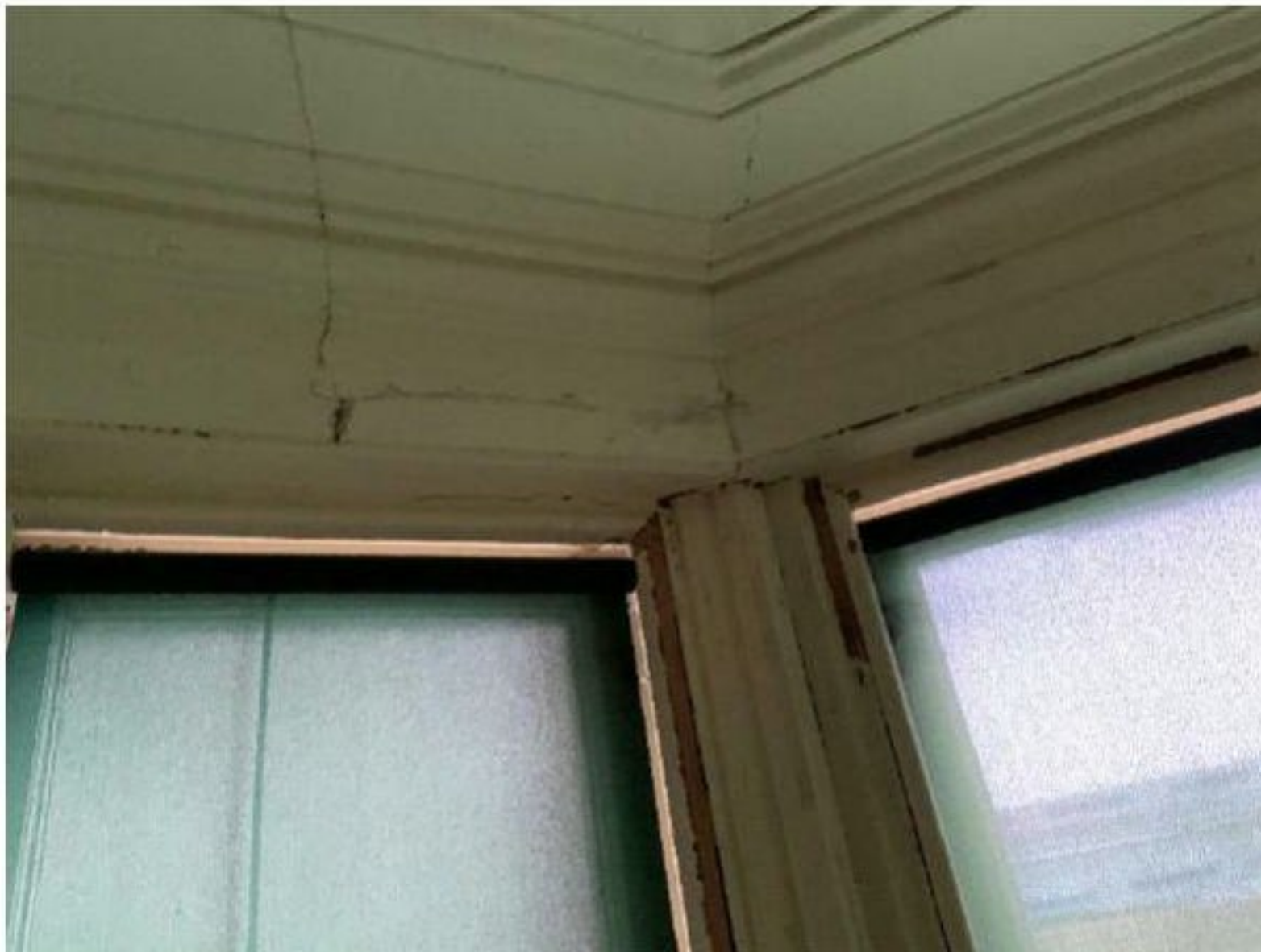
Photograph 1.11 Managers House - Internal Wall – Bay Window Cracking
