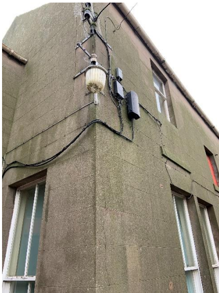
Photograph 2.11 America Street Offices - Quadrangle External Elevation – Section 2b – Corner Crack
