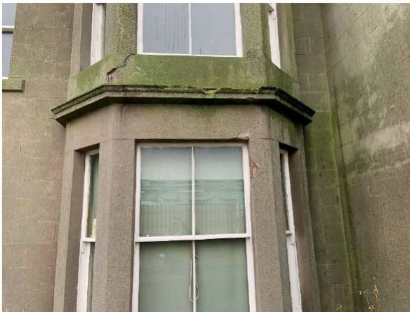
Photograph 1.03 Managers House - External Wall - Crack 2
