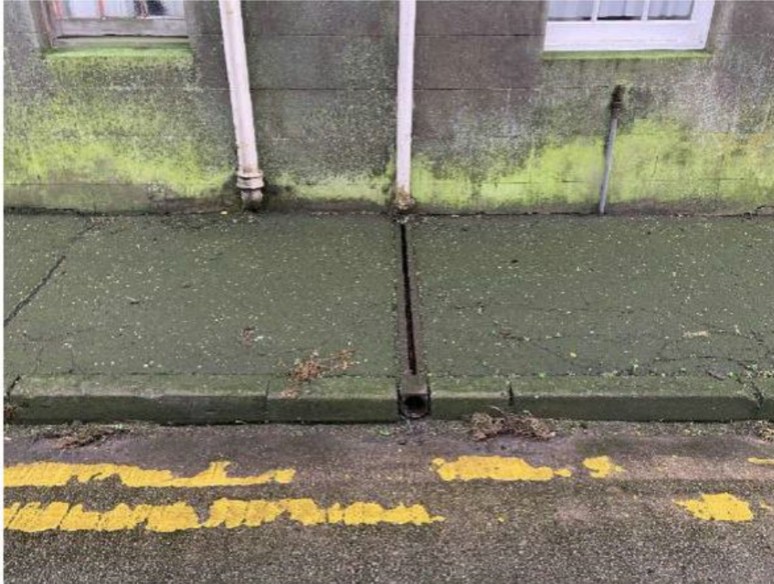
Photograph 1.04 Managers House - External Wall – Gable Drain
