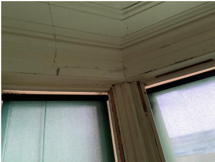
Photograph 1.11 Managers House - Internal Wall – Bay Window Cracking
