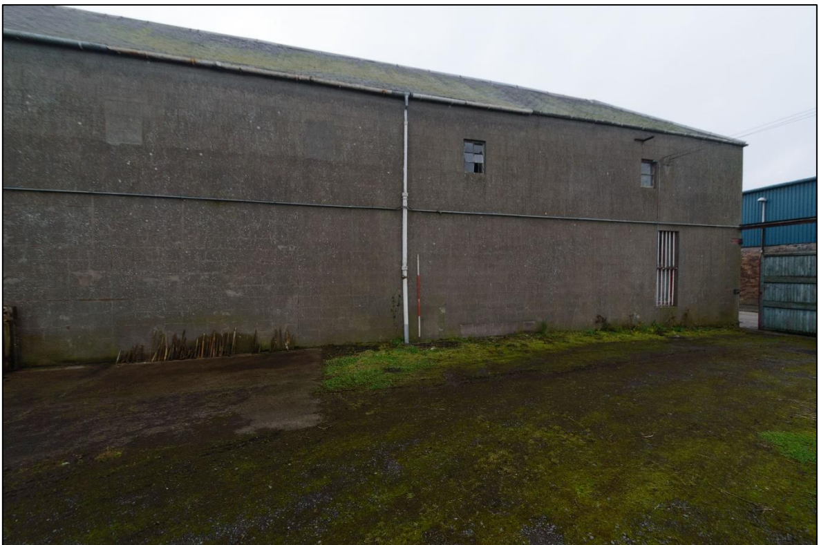
Illus 11 General view of NE elevation, adjacent to lots comprising 1 & 2 America Street.
