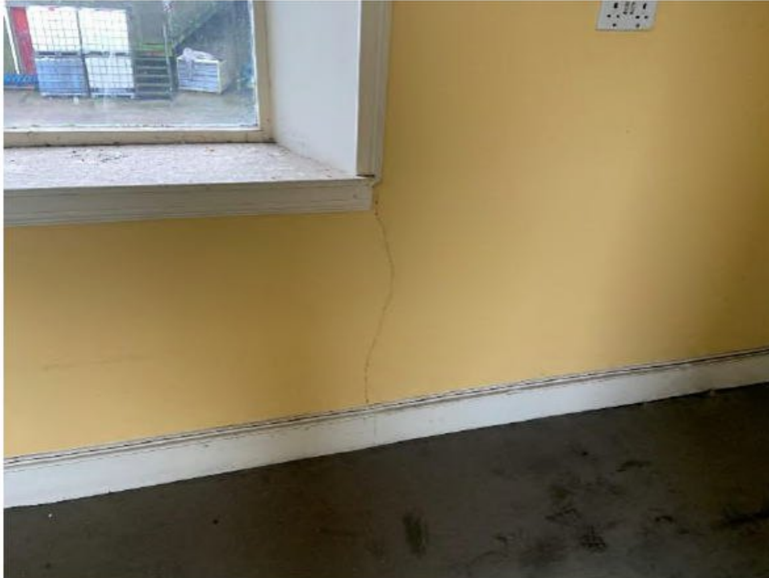
Photograph 2.14 America Street Offices – Internal - Cracks
