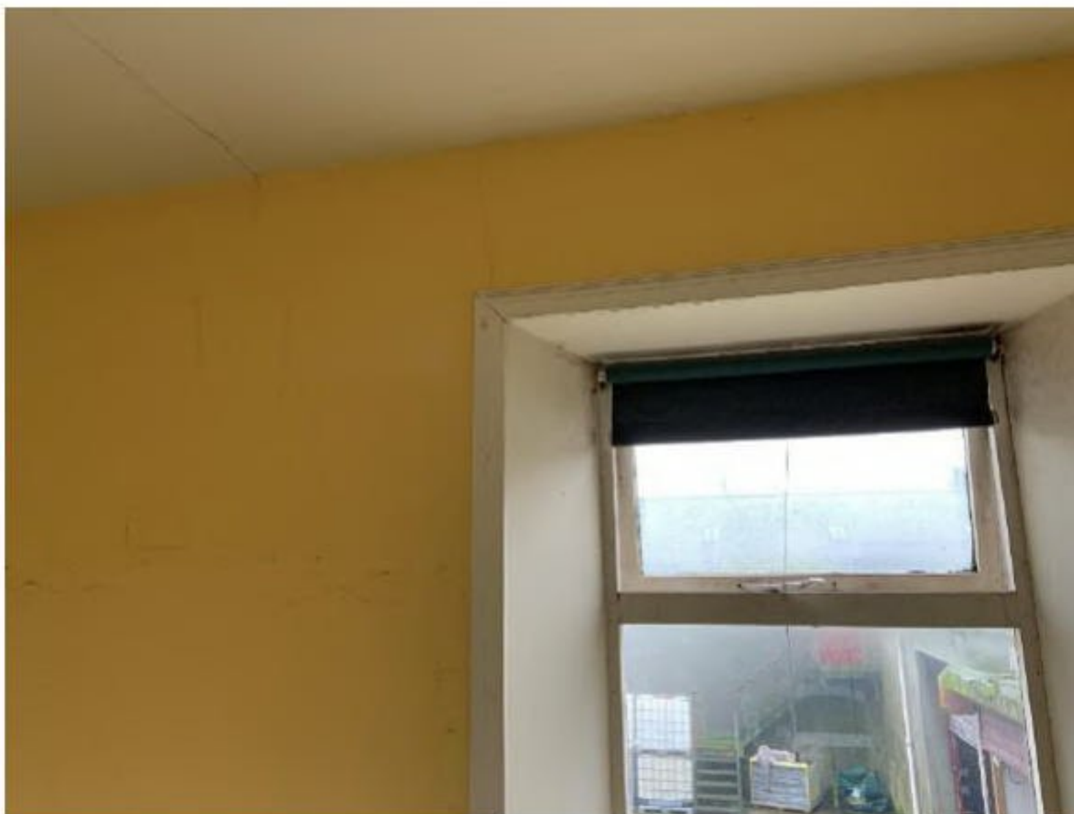
Photograph 2.13 America Street Offices – Internal - Cracks
