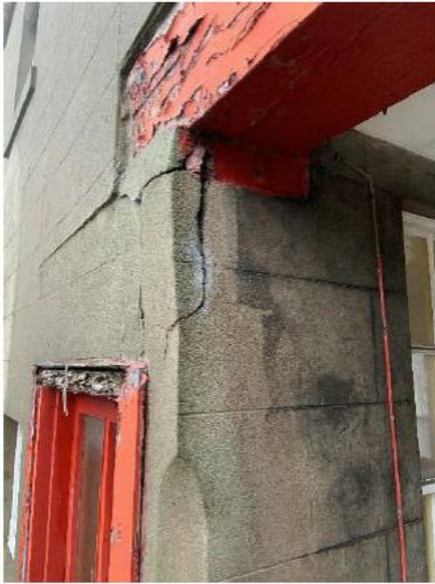
Photograph 2.08 America Street Offices - Quadrangle External Elevation – Arch Lintel Support
