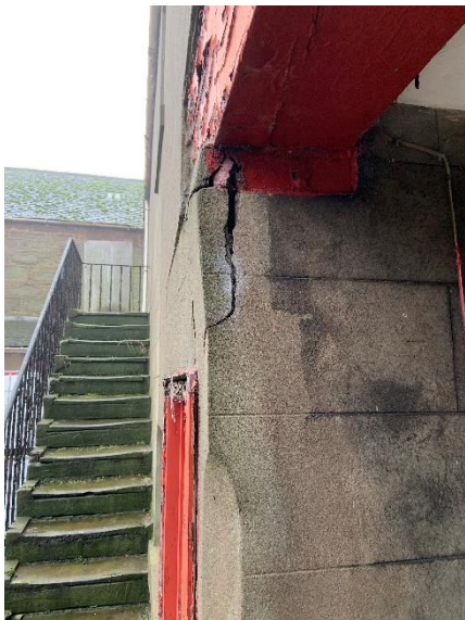
Photograph 2.09 America Street Offices - Quadrangle External Elevation – Arch Lintel Support
