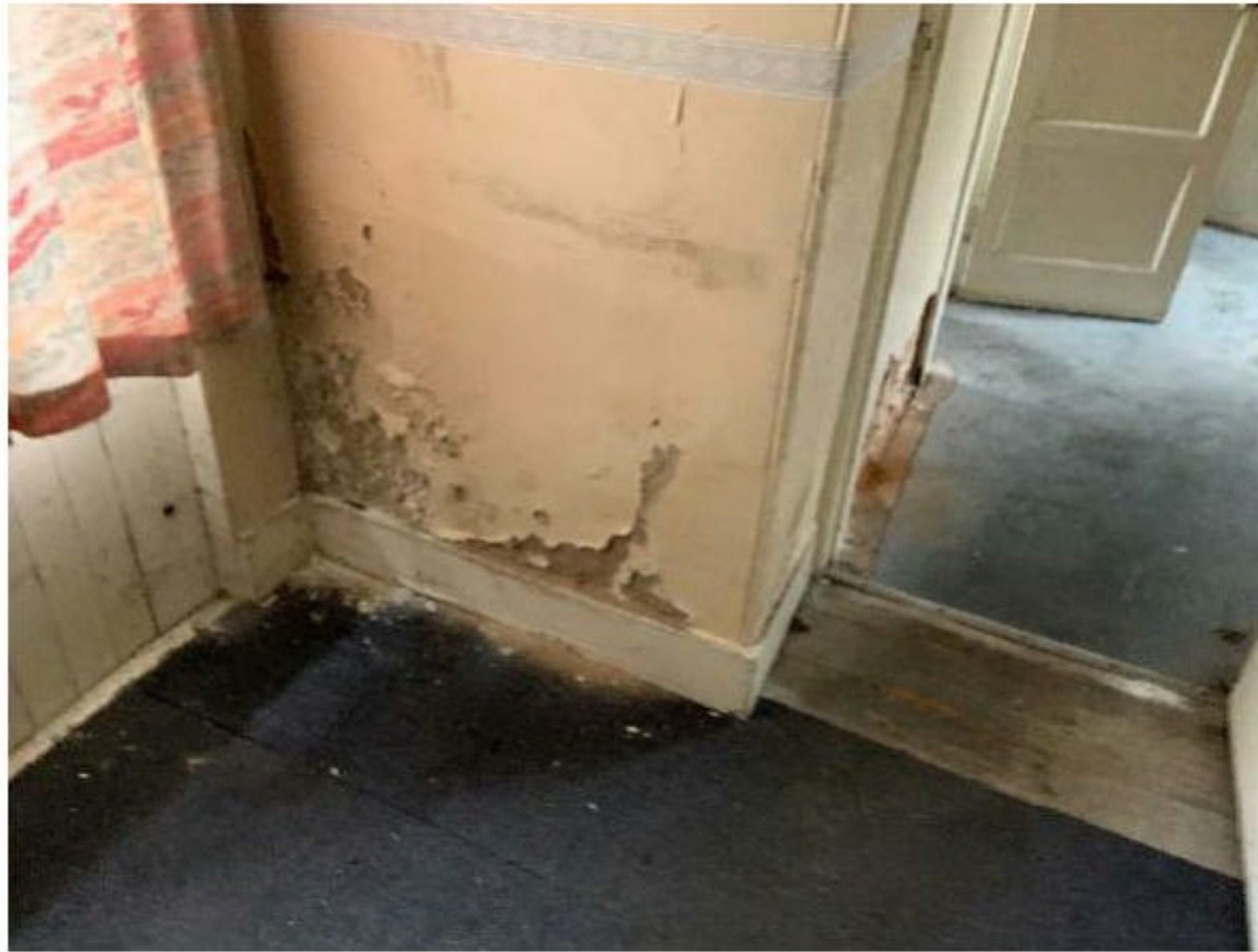
Photograph 1.08 Managers House - Internal Wall Dampness
