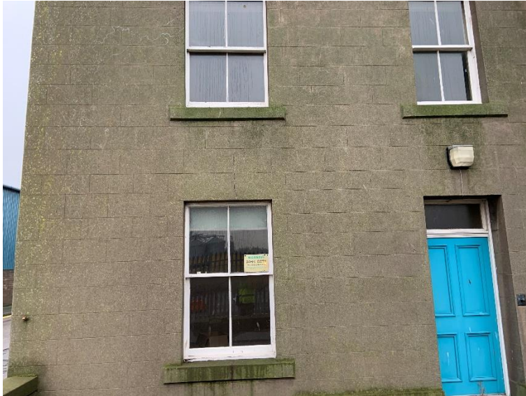
Photograph 1.02 Managers House - External Wall - Crack 1
