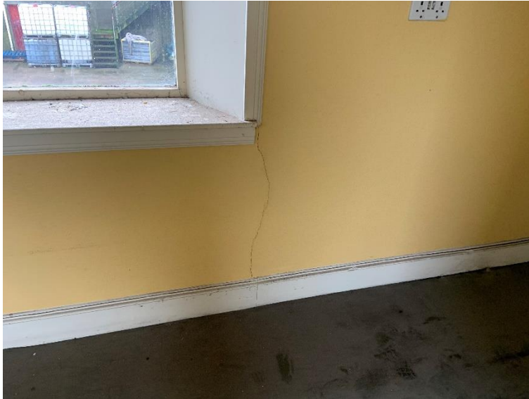
Photograph 2.14 America Street Offices – Internal - Cracks
