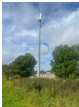
EE Mast at the top of Victoria Street
