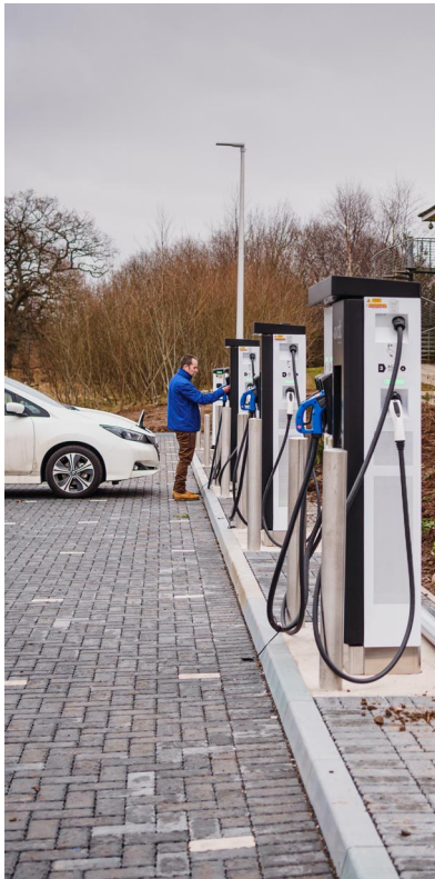
Electric vehicle charging points at Orchardbank in Forfar
