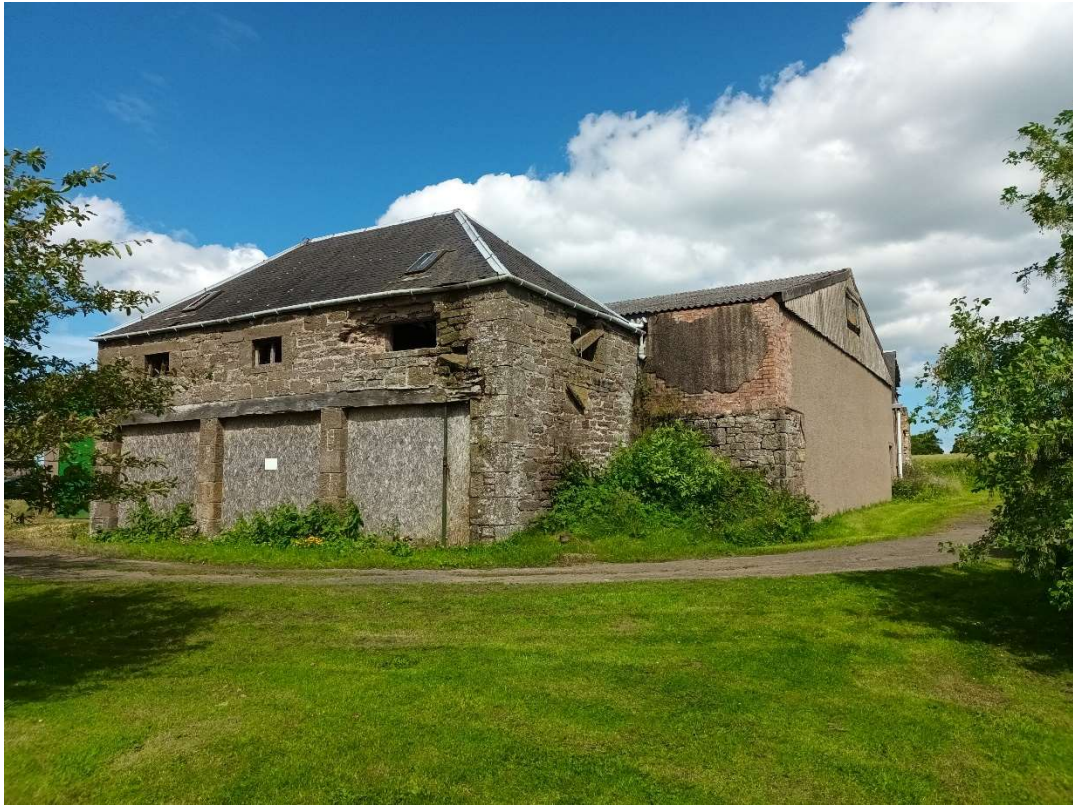
Appendix 4: Dilapidated farm range to the East of the Site
