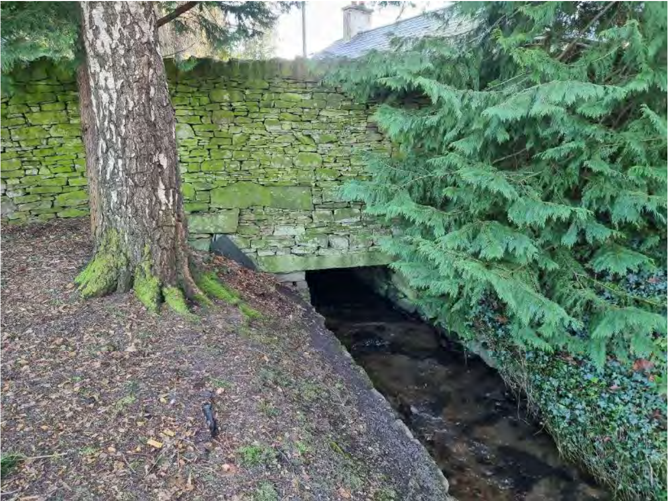
Photograph 1 – downstream end of the culvert which runs under the driveway of Dalnaglack. This photograph shows the Newtyle Burn as it enters the grounds of Burnbank.
