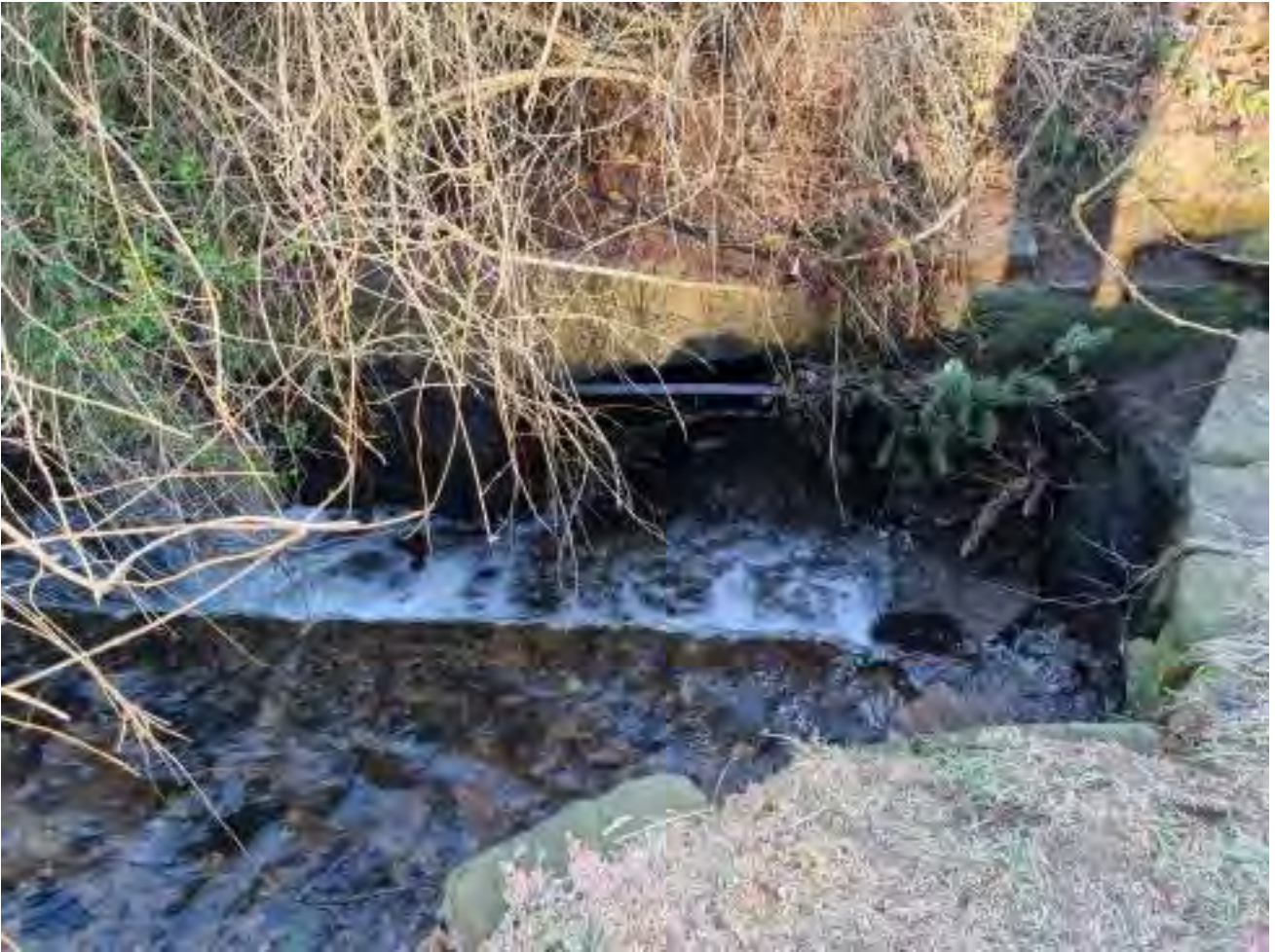
Photograph 5 – a view of the upstream end of the culvert which runs beneath Knox Close.
