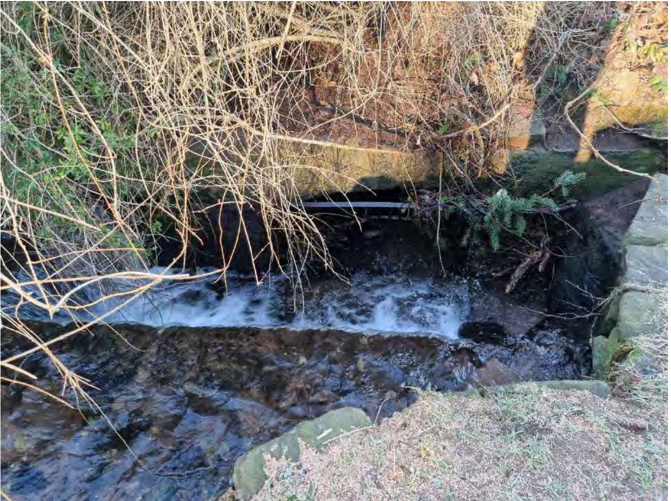
Photograph 5 – a view of the upstream end of the culvert which runs beneath Knox Close.
